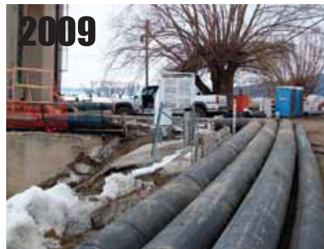
Grace, ID , CRS over concrete, industrial nightmare. RATING = CRN5
