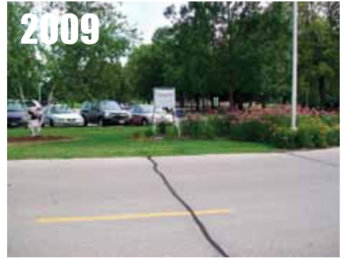
Milwaukee, WI , nearby road. RATING = CRN4
