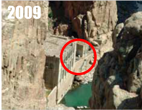
Buffalo Bill Dam, WY , sited on concrete, between two buildings. RATING = CRN5
