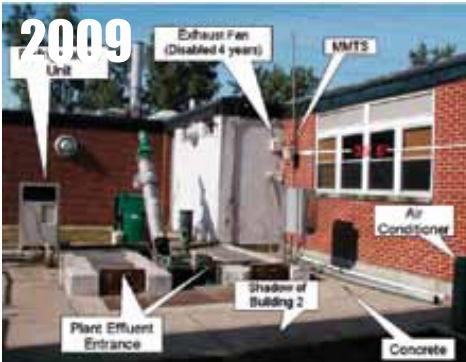
Urbana, OH , at city WWTP, mounted on brick wall, other multiple violations (see labels). RATING = CRN5
