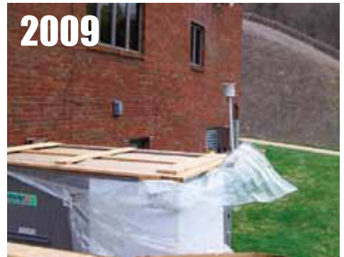
Williamsburg, KY , next to brick building (note the adjacent exhaust vent). RATING = CRN4
