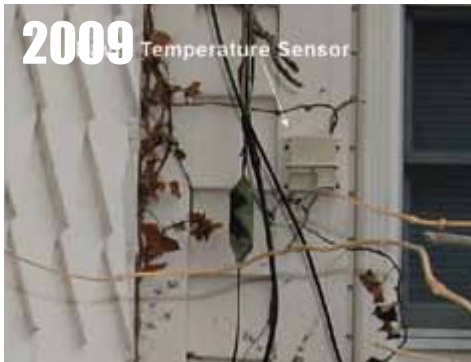
Tuckerton, NJ , unshielded sensor attached to building. RATING = CRN5
