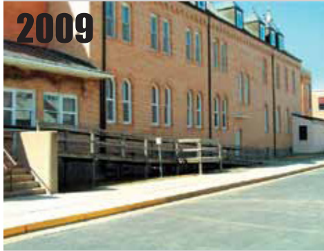
Richardton Abbey, ND , at edge of sidewalk, nearby road, building. RATING = CRN5
