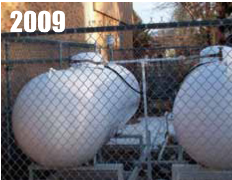
Dillon, MT. , at power plant building, sited on concrete border of sidewalk 6' from brick wall. RATING = CRN5
