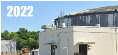
Same location at WWTP, but NWS reports: "MMTS MOVED 102 FEET SOUTHEAST." However, new site on rooftop is just as bad if not worse than original siting. Note exhaust fan nearby. RATING = CRN5
